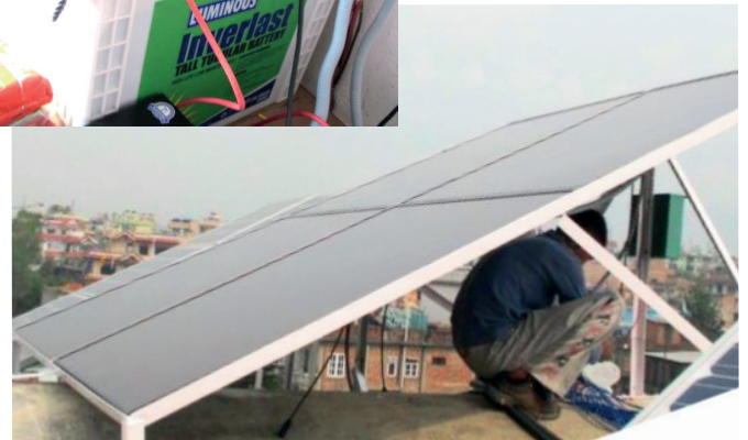
We rely heavily on solar power at Ghar Sita Mutu. Machteld Price made it possible for us to significantly upgrade our system.
