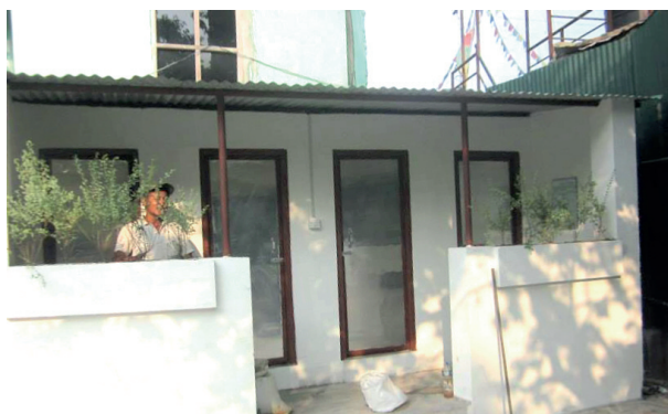
These are the new toilets at the Shangri-La School, which will significantly improve the comfort and hygiene for girls.
